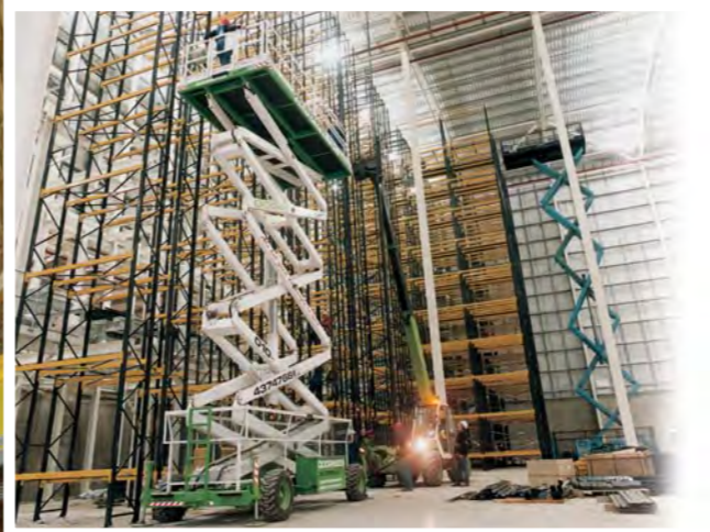
Link 51 installation teams use specialist skills, equipment and techniques to ensure racking is assembled safely and efficiently.
